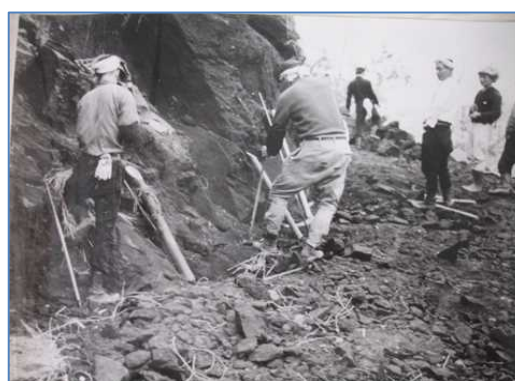
Photo 29: Construction work on a mountainside irrigation canal in the Site (Source: Midori Digital Archives)
